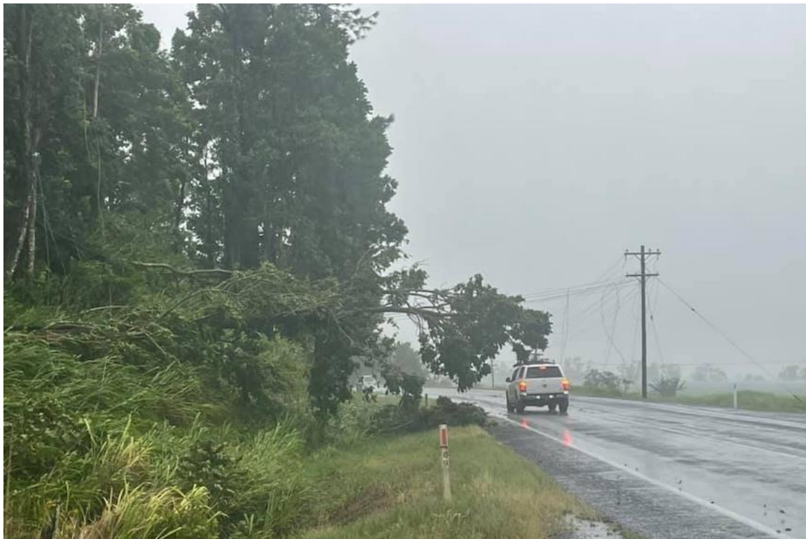
Figure 2.d. Power lines down on highway north of Codfish Creek in north Queensland. 25
