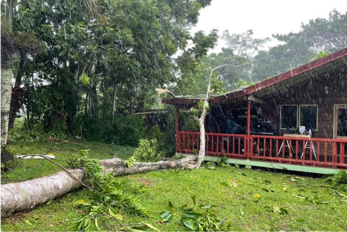
Figure 2.c. A tree falls onto the roof of a Mena Creek house in North Queensland on Monday. 24
