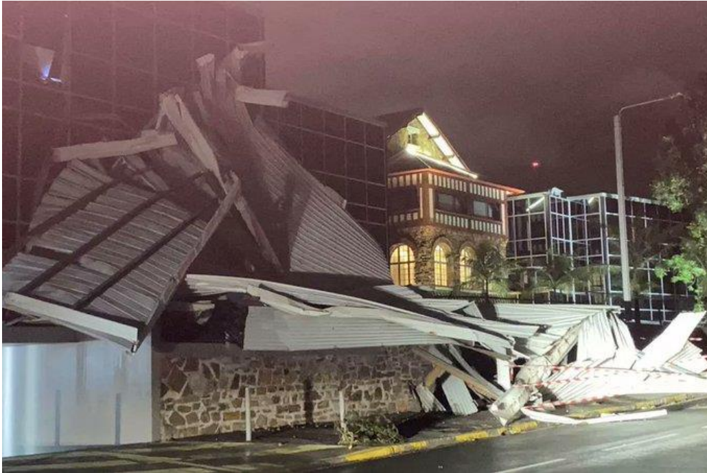
Figure 1.a. Pointe de l'Artillerie, the roof of the Portalis building crashed into the building opposite it. 19
